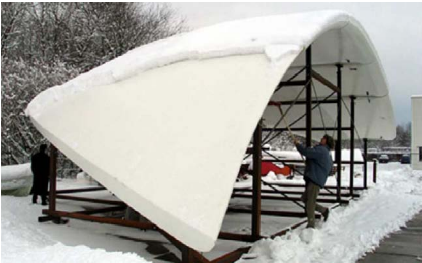
Fig. 41-42. Roof segment (left) and fitting of all the roof segments of the lower wing of 'The Library' at Holland Composites in March 2005.
