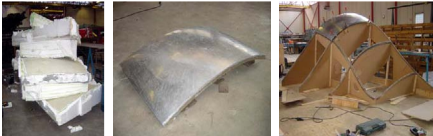
Fig. 8-10. Left over polystyrene moulds used to make negative concrete moulds (left), exploformed aluminium panel (center) and fitting of a panel on a wooden fitting mould (right).
