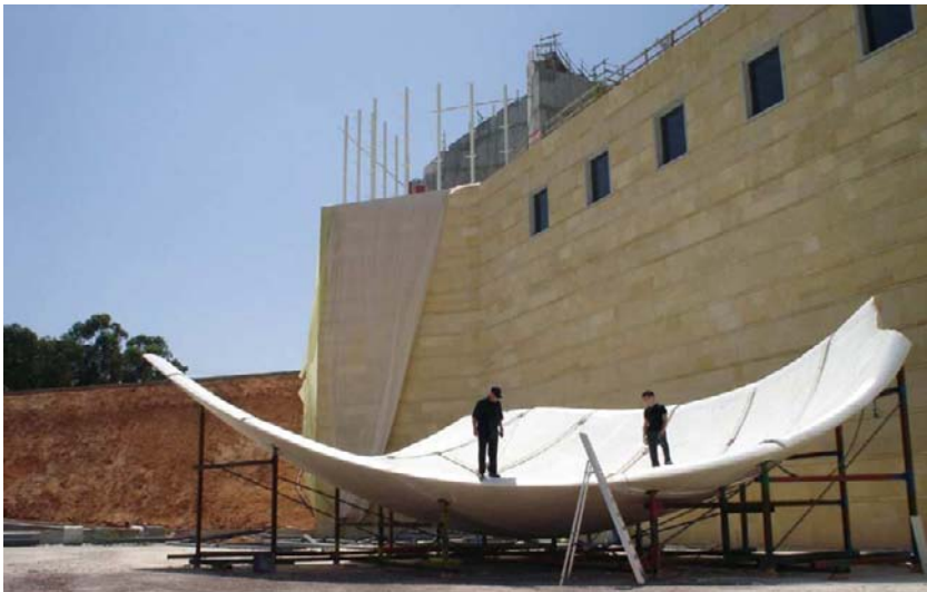
Fig. 48-49. Assembly of the roof segments by gluing and bolting glass fibre polyester plates on the seams before applying the finishing layer
