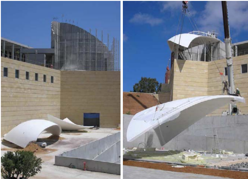
Fig. 46-47. Preparation and hoisting of the upper and lower wing of the Library in August 2005
