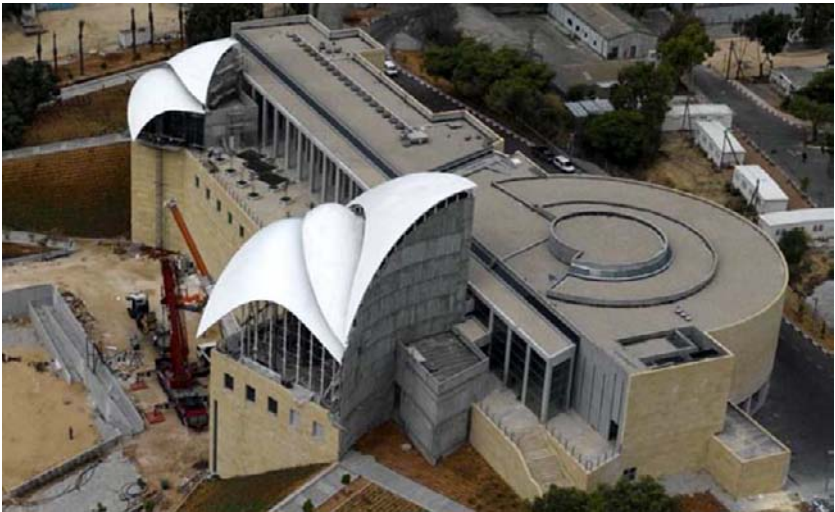
Fig. 50-51. View of the building site on the 6 th of November 2005, photographed by Ardon Bar Hama.
