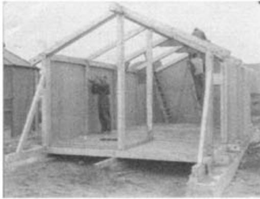
7.5 A four-bay ANARE Mark 1 building being erected. This is the second time it was erected as they were test-erected in Melbourne prior to departure
