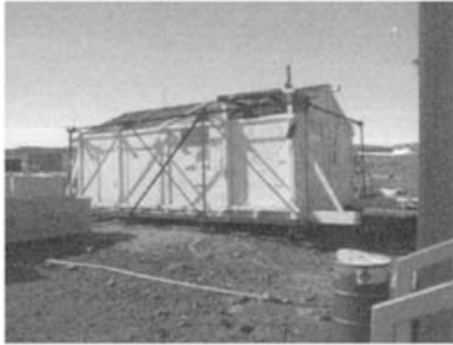
7.8 The Mawson ANARE Mark 1 Met/Tech buildings packed ready to return to Australia
