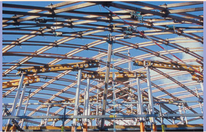
Support scaffolding and the gridmat midway through the forming process, showing the telescoping scaffold system in action.
