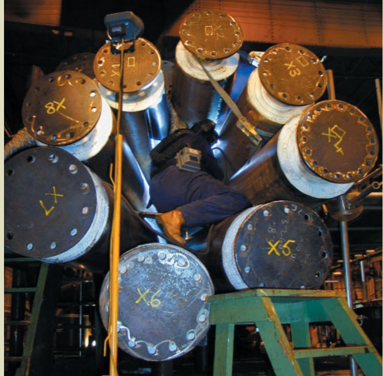
Figure 6: Specials. Some of the welds required left-handed welders using modified welding equipment, simply to get at the more 'embedded' welds.
