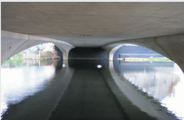
The in-situ reinforced concrete soffit of Ballingdon Bridge, including bat boxes. The in-situ concrete ties the precast concrete unit together to form an integral structure.
