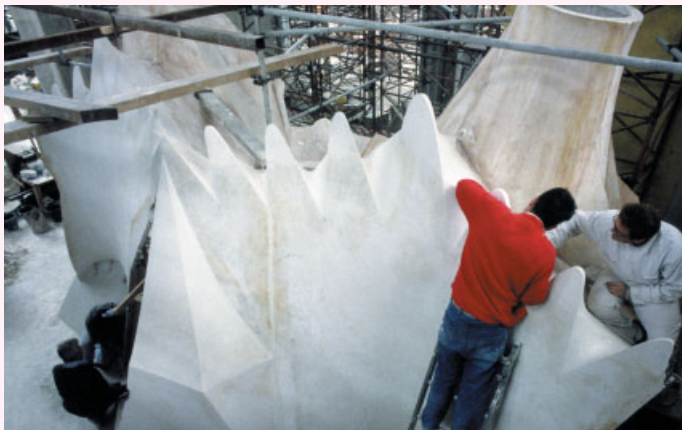
Full-scale mould-master for part of the central nave ceiling vaults (inverted for convenient fabrication at ground level). This plaster of Paris mould-master is for the production of fibreglass production moulds for building components.
