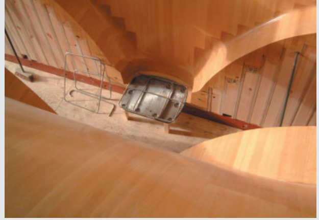
The 'foot' of the Ballingdon Bridge pier mould split at Buchan's works in Lancashire, ready for installation of the reinforcement.
