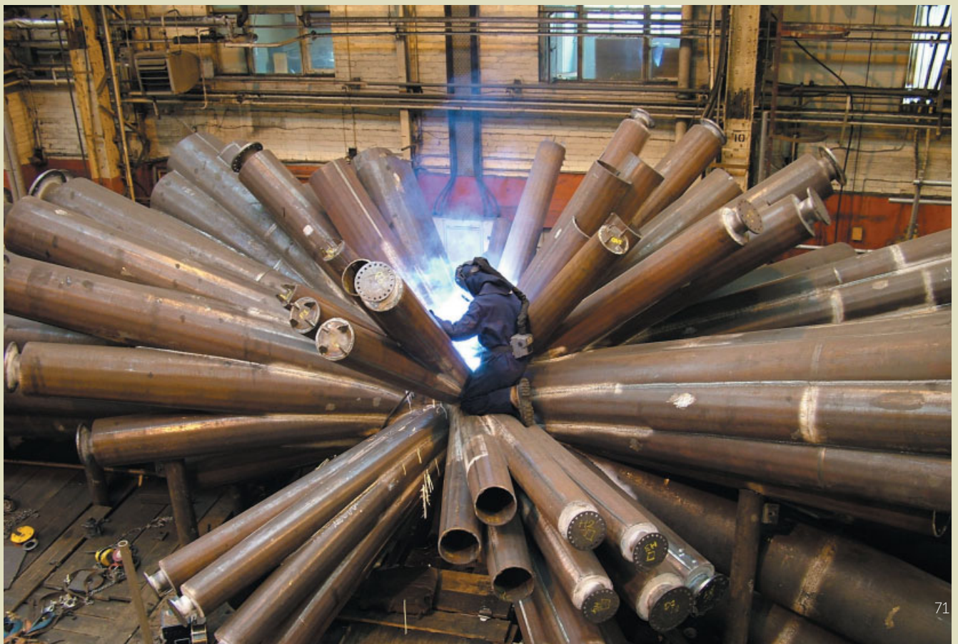
The contorted geometry of the core required bespoke tooling and dexterous hands.
