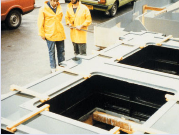
A prototype one-piece GFRP form for the beam grid of the Lloyd's Building. It was designed to be withdrawn upwards to avoid having the downward tapered beam profile of a conventional waffle floor.
